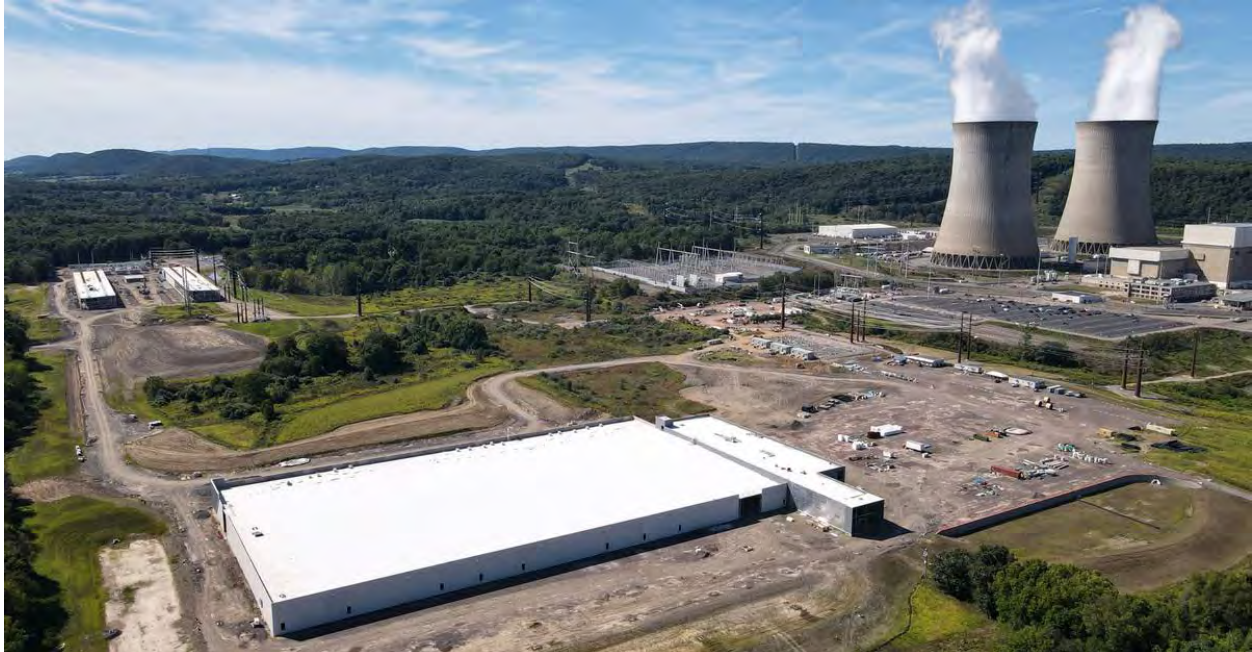
The first building at Talen Energy subsidiary Cumulus Data's nuclear-powered Susquehanna data center campus in Pennsylvania [photo: Talen-Cumulus]
